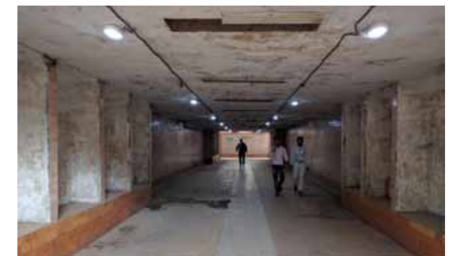
Poor maintenance, unclean floors, poorly lit passage-way
