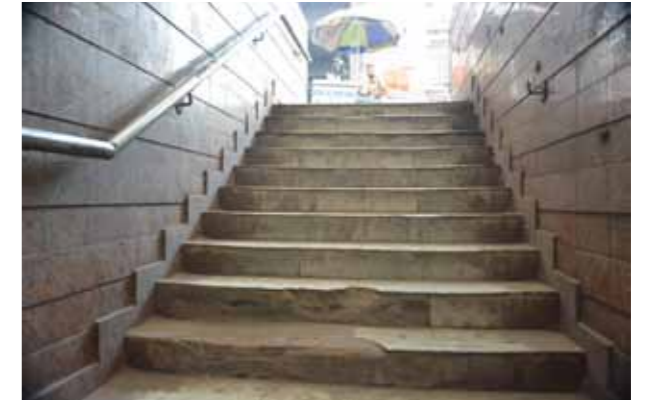
Missing handrail & broken staircase
