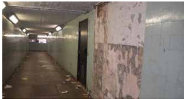
Ill-maintained subway before renovation
