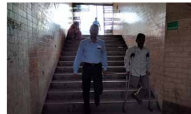
Absence of handrails
