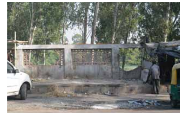
Broken boundary wall
